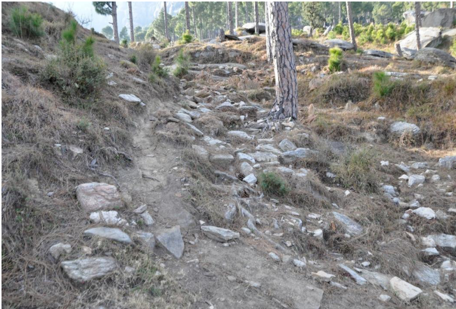
Fig. 18 - One of the damaged stairway at steep places of the site.
