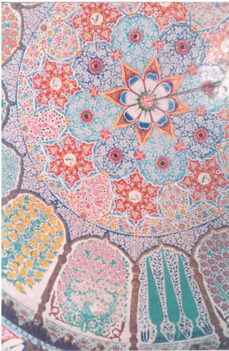
Pl. II. (Kohat): Shaikh Allah Dād Tomb, showing painted decoration in polychrome soffit of the dome
