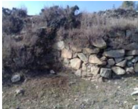
Fig. 5- wall remains in dilapidate condition.
