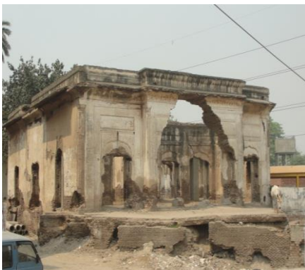
Fig. 4 - Front facade showing missing brick masonry.
