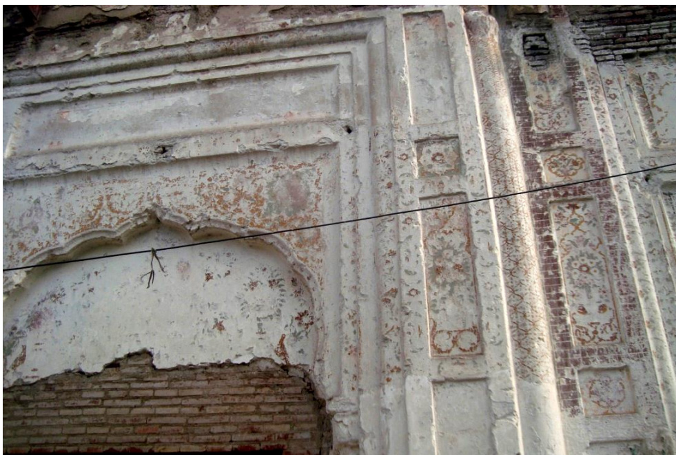
Fig. 6 - Facial decay and deterioration.
