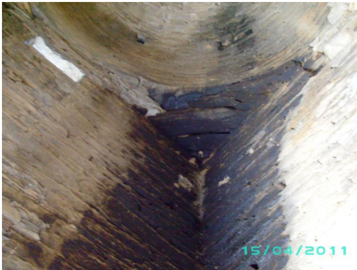
Pl. 7: Balo-Kale Gumbat: Interior detail of the south-eastern corner (before conservation) showing three parallel wooden architraves over which the projected cornice moulding is placed
