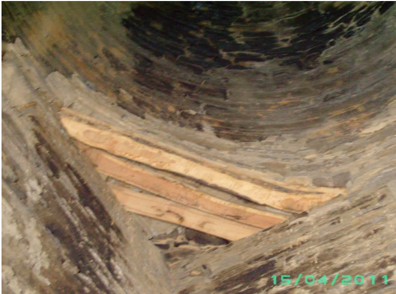
Pl. 8: Balo-Kale Gumbat: Interior detail of the south-western corner showing three parallel wooden beams over which the projected cornice moulding is placed (after conservation)
