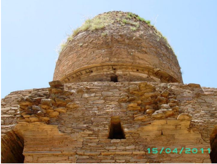
Pl. 6: Balo-Kale Gumbat: View from the eastern side showing series of supporting brackets to the dome.
